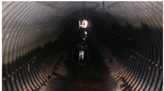
Compromised 90" Corrugated Metal Pipe
