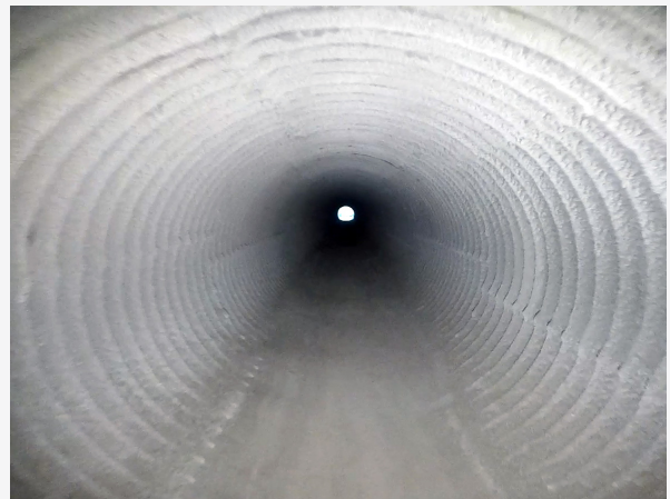
Post installation inspection of the GeoKrete lined culvert shows precision and cleanliness of the application.
