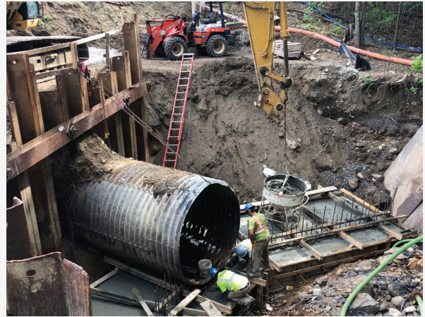
NHDOT culvert required significant reinforcement as part of the entire rehab process.
